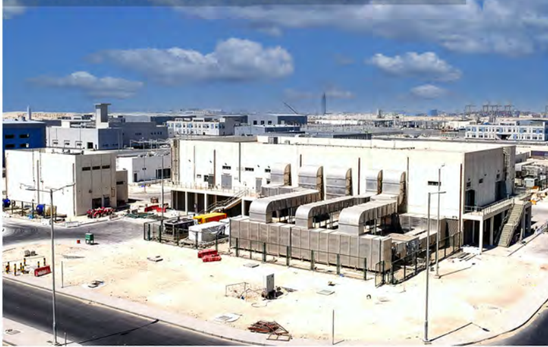
NPP 0050 New Port Project QENFB Infrastructure, Roads & Utility Buildings: DI Covers for Underground Utilities
